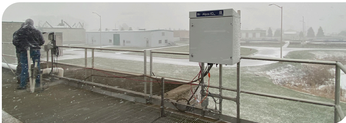
Outdoor Alyza IQ PO4 analyzer installed at the aeration outlet channel, providing real-time orthophosphate measurements to SCADA.
