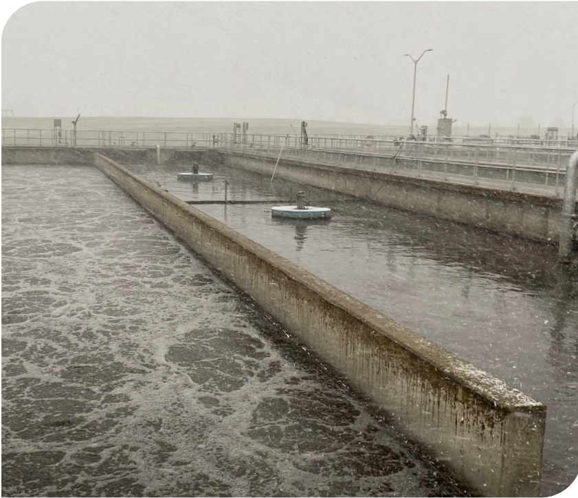
3-pass activated sludge system at Fond du Lac WRRF. Pass 1 (ORP controlled) and Pass 2 (ammonium controlled) shown.
